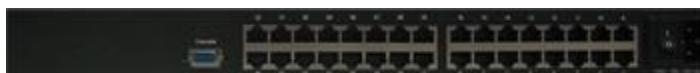
Close up of the Rear View of Cat-6 KVM showing Qty 16 RJ45 interface Ports
