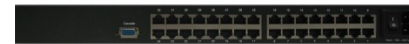
Close up of the Rear View of Cat-6 KVM showing Qty 32 RJ45 interface Ports
